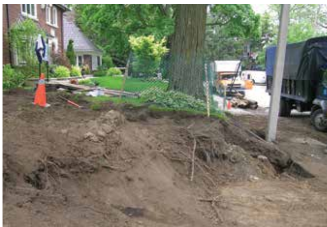
Roots of mature trees have been severed during construction.
